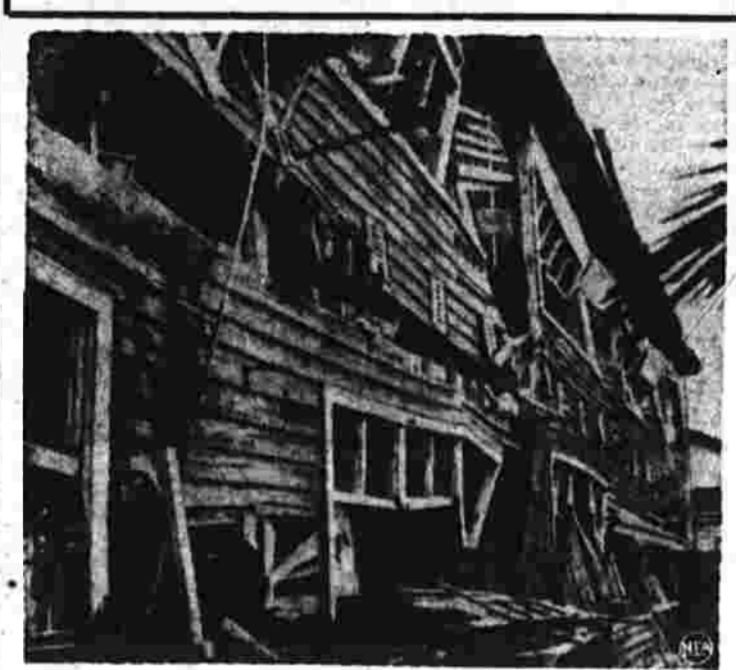
Mile and a half away: This wood-frame building, 8,000 feet from point of blast at Nagasaki, was badly ruptured. Maximum distance for property damage would be about five miles.
